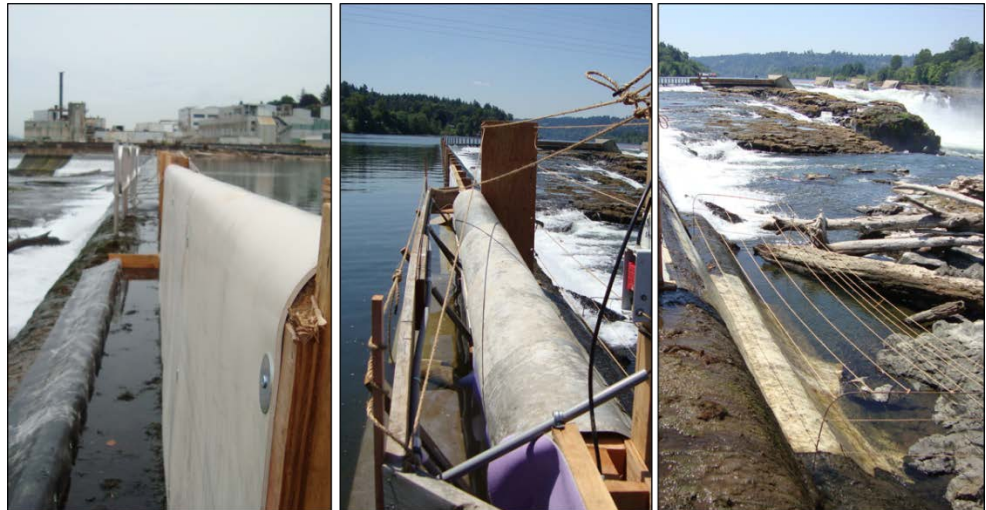
Figure 2. Rubber faced lamprey ramp and resting pool curb (left), debris “cattle guard” (center), and epoxy coated concrete and avian deterrent (right).
